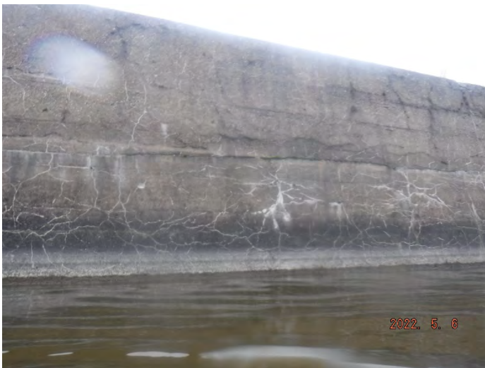
Typical Map Cracking with Efflorescence at Pier
