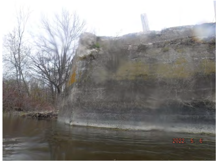
Map Cracking/Spalling at East Abutment
