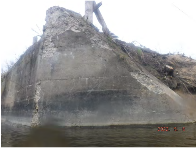
East Abutment South Wingwall Deterioration
