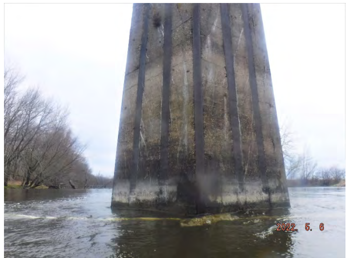
Upstream Nose of Pier Vertical Cracks
