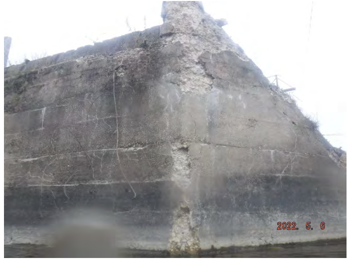
East Abutment South End Spalling
