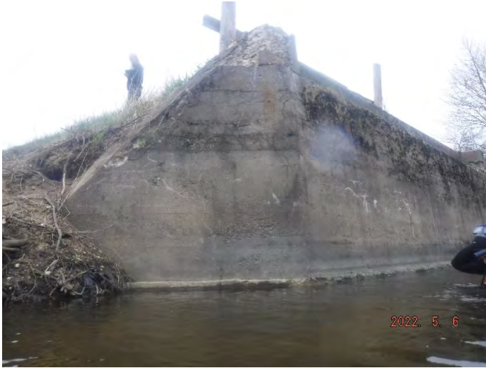
West Abutment South Wingwall Deterioration
